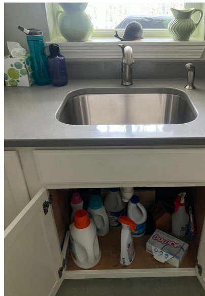
Mudroom faucet susceptible to pipes freezing
