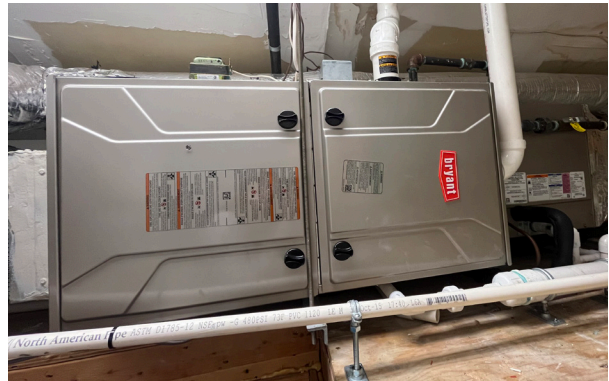
HVAC system in the attic (propane system)
