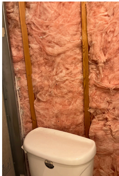
Moisture noticed in bathroom sheathing and insulation
