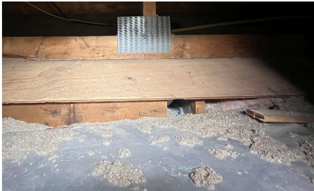
Additional attic insulation recommended
