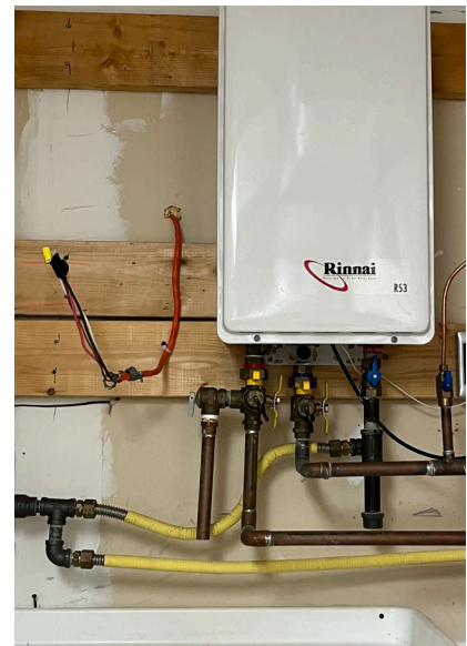
Rinnai on-demand hot water heater (propane system)
